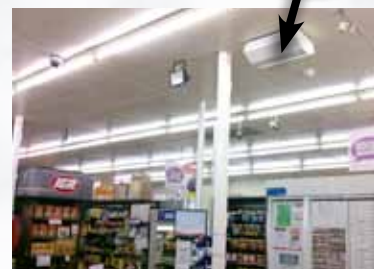
PROTECTION: The PROTECT Fog Cannon installed at David Wilkes' Beaconsfield IGA
